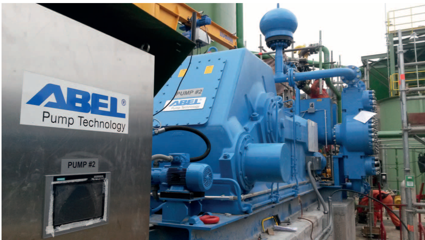
The ABEL HMQ piston-diaphragm pump was installed and commissioned in mid-August 2015 at the Latin America underground silver mine and has been in continuously operation since
