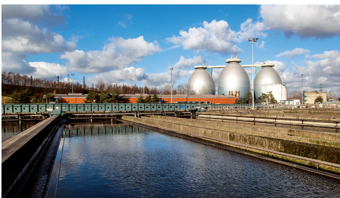
Fig. 1: ABEL pumps have been in use at the central sludge treatment of EMSCHERGENOSSENSCHAFT in Bottrop for years where they have proved to be successful (Source: Emschergenossenschaft Essen)
